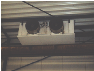
Evaporator drip tray
